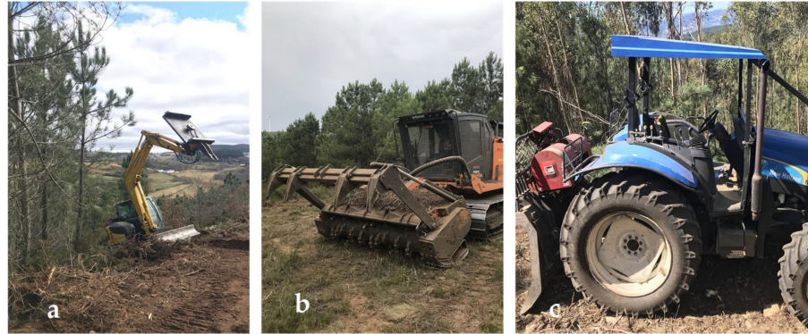
Figure 2. Excavator with a shredder head (a), forest shredder (b), tractor with a crushing implement (c).
