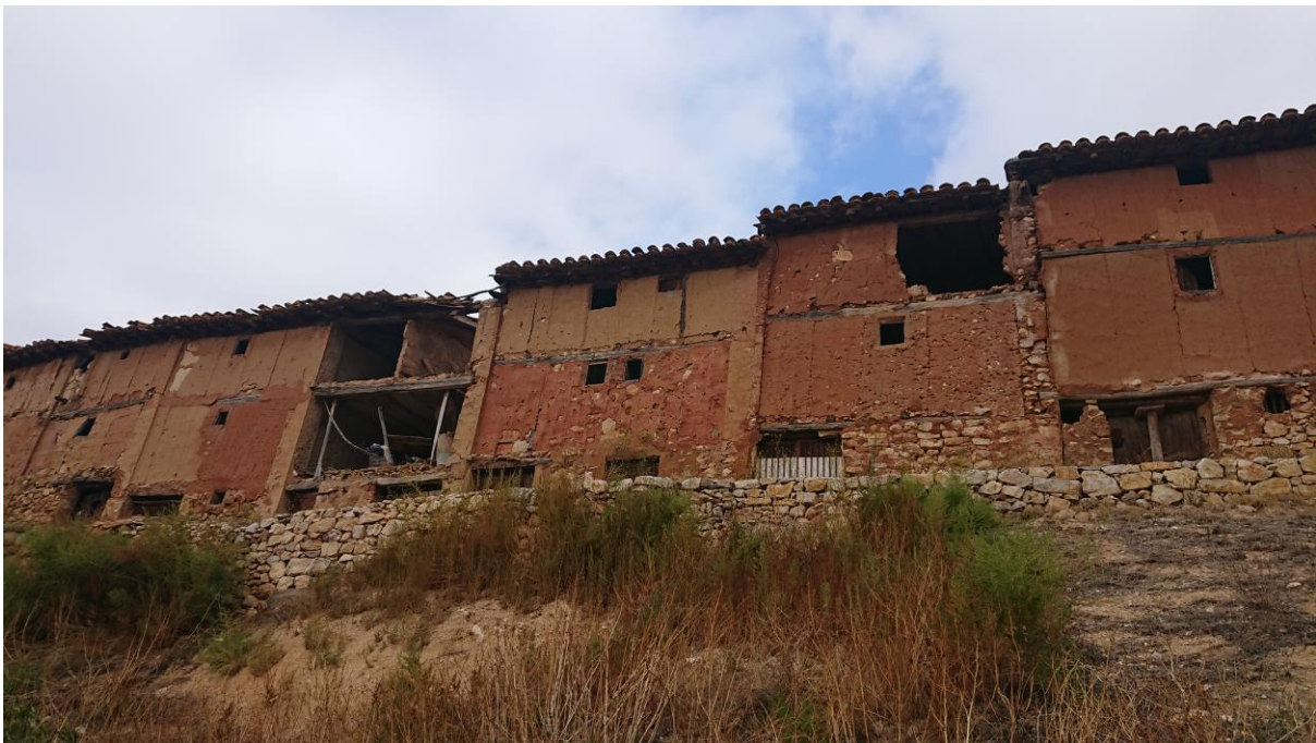
Figure 15. Empty vernacular dwellings in a poor state of conservation located on Calle del Barranquillo, Casas Bajas, 2021. Author: Eva Tortajada.
