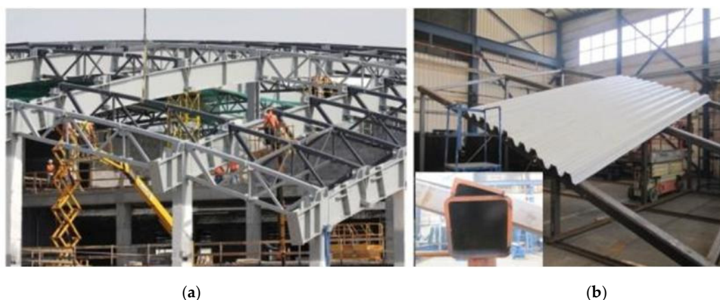
Figure 15. Two steel structural systems supporting transformed folded sheets by Żwirek [38]: (a) the erection of the final shell roof; (b) experimental tests.
