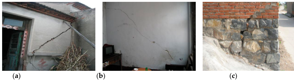
Figure 1. Surface walls and foundation damage above the mining area. (a) Wall cracking. (b) Cracks in the wall. (c) Basic cracking.
