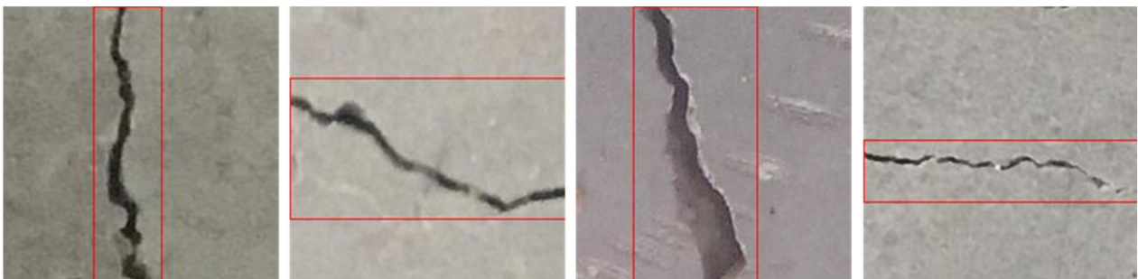
Figure 9. Detection results of the concrete surface cracks.
