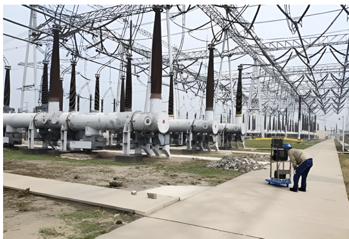
Figure 7. The photo of PD signals field acquisition process at a GIS substation.
