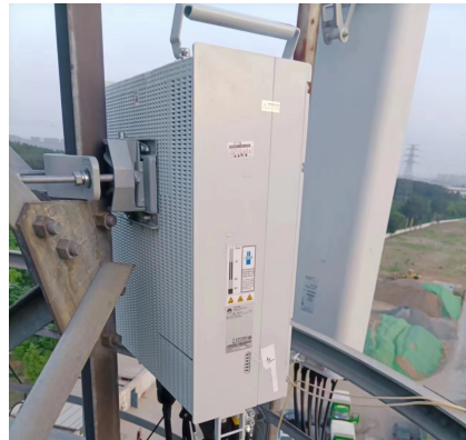
Figure 5. RRU installed on the tower, adjacent to the antenna.
