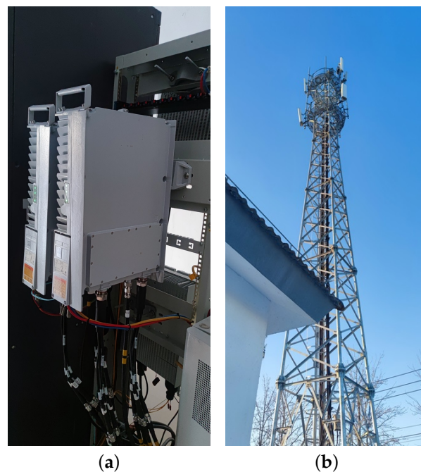
Figure 4. 5G-R RRU equipment and antenna. (a) 5G-R RRU equipment. (b) Base station feeder and antenna.
