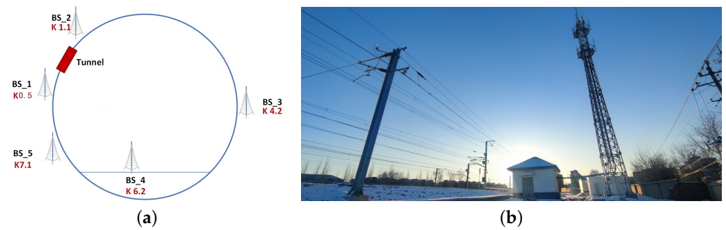
Figure 3. Locations of on-site equipment rooms and base station towers. (a) Locations of 5G-R Base Stations. (b) On-site equipment room and base station tower.
