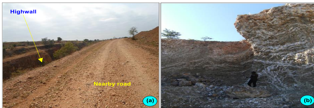
Figure 6. (a) An illustration of the close location of the excavation to the access route and Frankie Mine, and (b) the unstable highwalls of the excavations at Nyala Mine.
