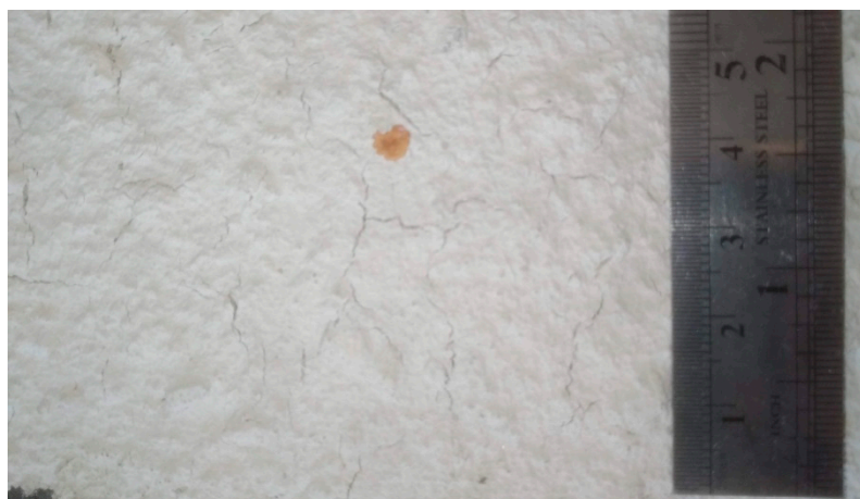
Figure 5. Detail of DG 1.0 D surface with microcracks.
