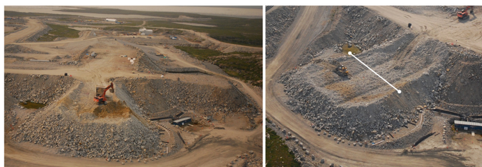
Figure 1. Overview of test piles area during initial stages of the Type I test pile deconstruction (left) and the Type I test pile at excavation of bench three with two sampling trenches (right). The white line on the right photo shows the approximate location of the 15 m profile. Photographs courtesy of Sean Sinclair.
