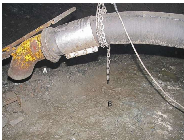
Figure 4. Approximately 0.3 m broken ore left on the drive floor before (A) and after (B) vacuuming. Supersucker hose diameter 200 mm.
