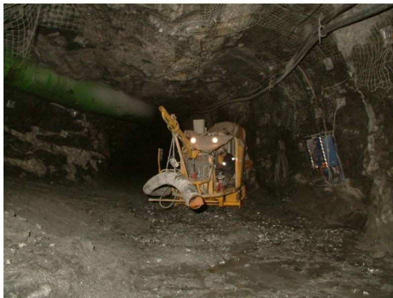
Figure 6. Ausvac Supersucker unit underground in an ore drive. The accumulation of broken ore residues on the drive floor in front of the Supersucker is clear.
