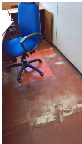
Figure 2. Example of damaged vinyl–asbestos floor tiles in office building.
