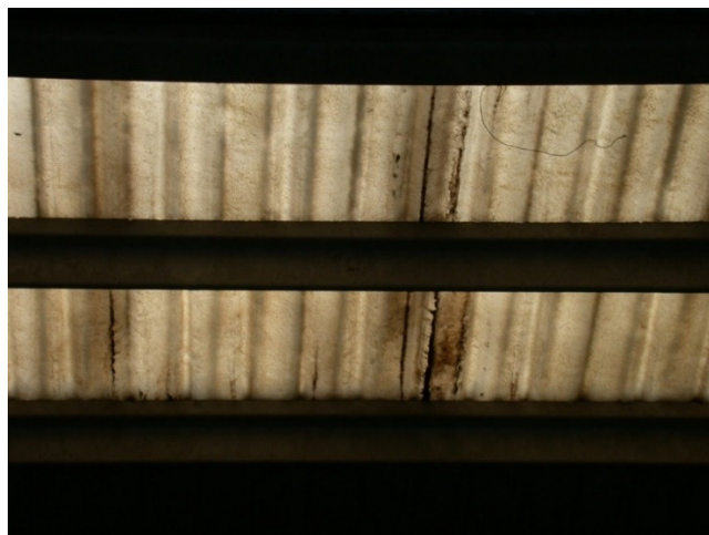
Figure 7. Example of a damaged exposed asbestos cement roofing in indoor environments.
