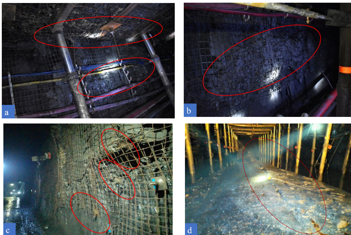
Figure 5. Failure characteristics of a strong mining roadway in RAR 23204: (a) stepped roof subsidence and mining sidewall failure; (b) failure instability of mining sidewall; (c) pillar sidewall failure instability and bolt failure; (d) severe floor heaving and floor cracking.
