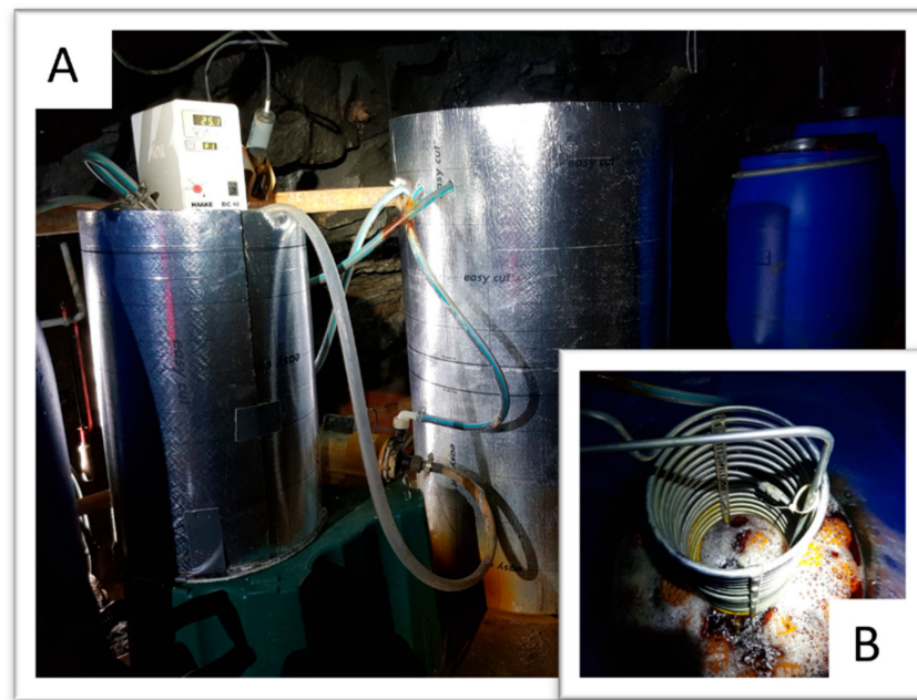
Figure 9. (A) Installed isolated 220 L bioreactor (right) with thermostat (left); (B) Close-up inside the bioreactor with heating coil and fine-pearled air in the bioleaching solution.
