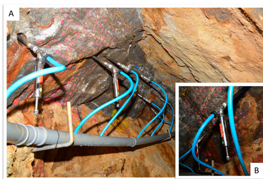
Figure 6. Bottom road at the testing site showing (A) the ore vein “Wilhelm Stehender Nord” with drainage boreholes and (B) a close-up of one of the drainage boreholes with installed back-pressuring valve.
