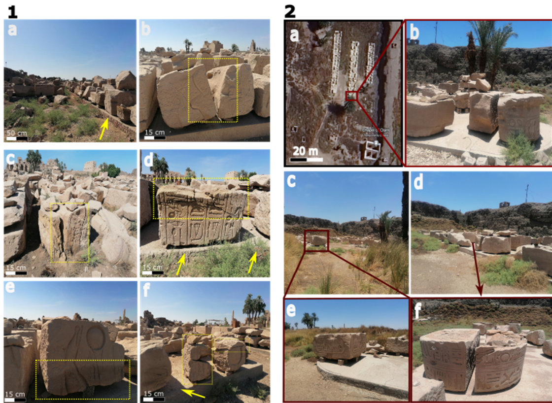
Figure 9. (1) and (2) Analysis of the mechanical impact of cumulative earthquakes and flooding events on the structures at Karnak. (1a) A general view showing scattered stone blocks, displaced due to mechanical forces, now resting on a loose red brick mastaba. (1b) Close-up of fractured stone blocks, illustrating the damage. (1c) Various stone blocks that have slid and become embedded in the soil, likely as a result of earthquake tremors or the impact of flooding waves. (1d–1f) Detailed views of mechanical chipping, fractures, and cracking observed on the stone surfaces, highlighting the extent of the damage. (2a) A Google Earth image of the study area, focusing on the northeastern part of Karnak, showing the current state of the stone blocks. (2b–2f) Documentation of various damage aspects of the stone blocks, including splitting, chipping, and fracturing, illustrating the ongoing deterioration of the site due to mechanical forces.
