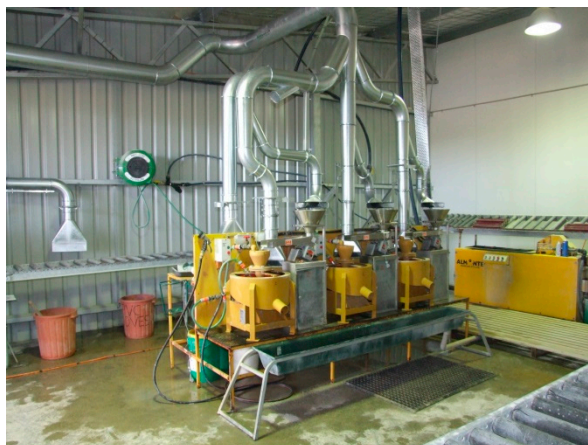
Figure 3. LGL gravity concentrator facility.
