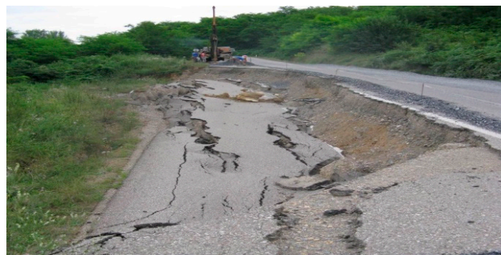
Figure 3. Slope on the section: Šabac-Tekeriš-Zavlaka at km 10 + 225 [24].
