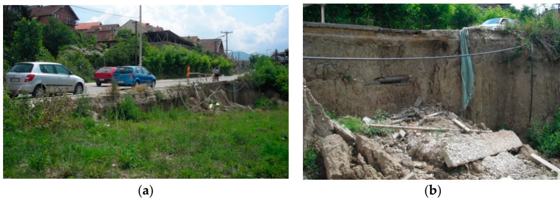
Figure 5. Slipway on the part of the regional road II of line R234, Novi Pazar-Rajetiće (a) right view; (b) central view [26].
