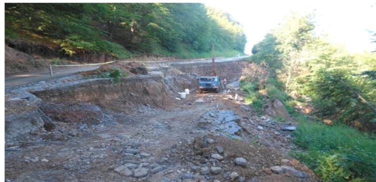
Figure 6. Formed slip on the part of the state road IIA-137 (P-127) [27].
