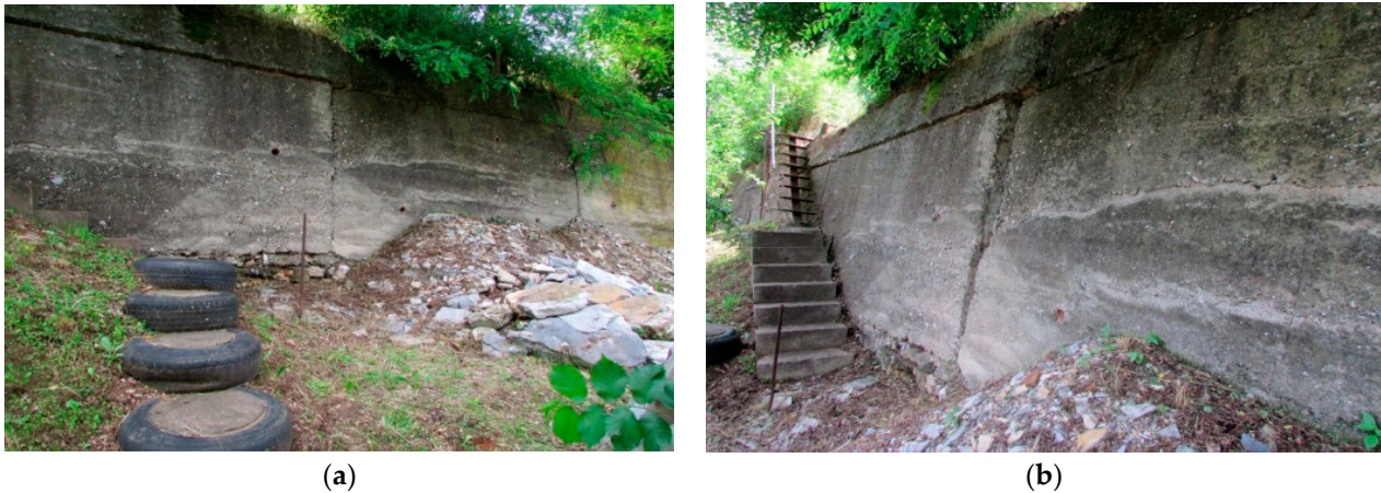
Figure 7. Details of the supporting wall in the basis of the road embankment at the site “Pejčina krivina” (a) right view; (b) left view [28].
