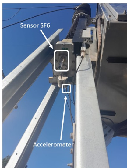
Figure 19. SF6 sensor and accelerometer installed in the pole crankcase.
