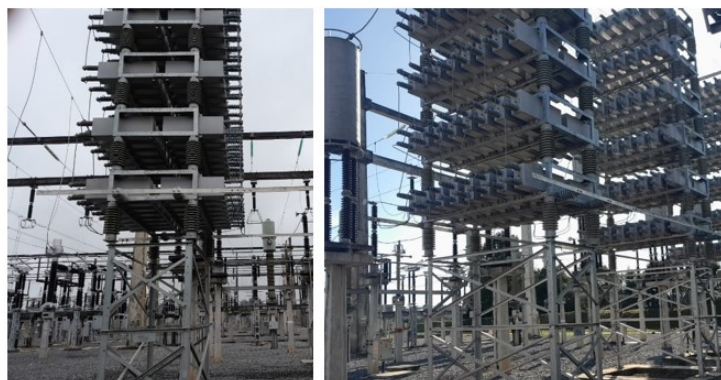
Figure 14. Bank of capacitors connected to the HVCB GL 314X.
