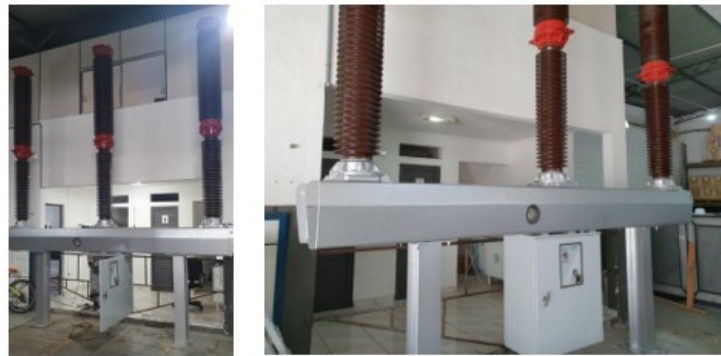
Figure 2. CGL 312 test circuit breaker.
