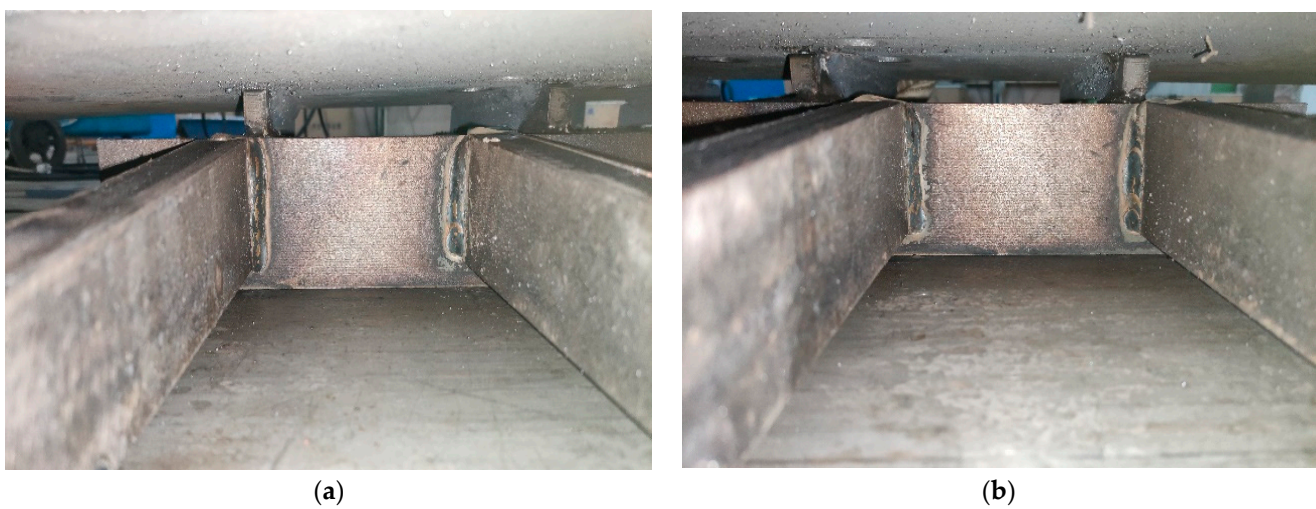
Figure 24. Welds of fixed comb plate and support system: (a) From top to bottom in Figure 22b, below the third teeth, (b) Below the fourth teeth.
