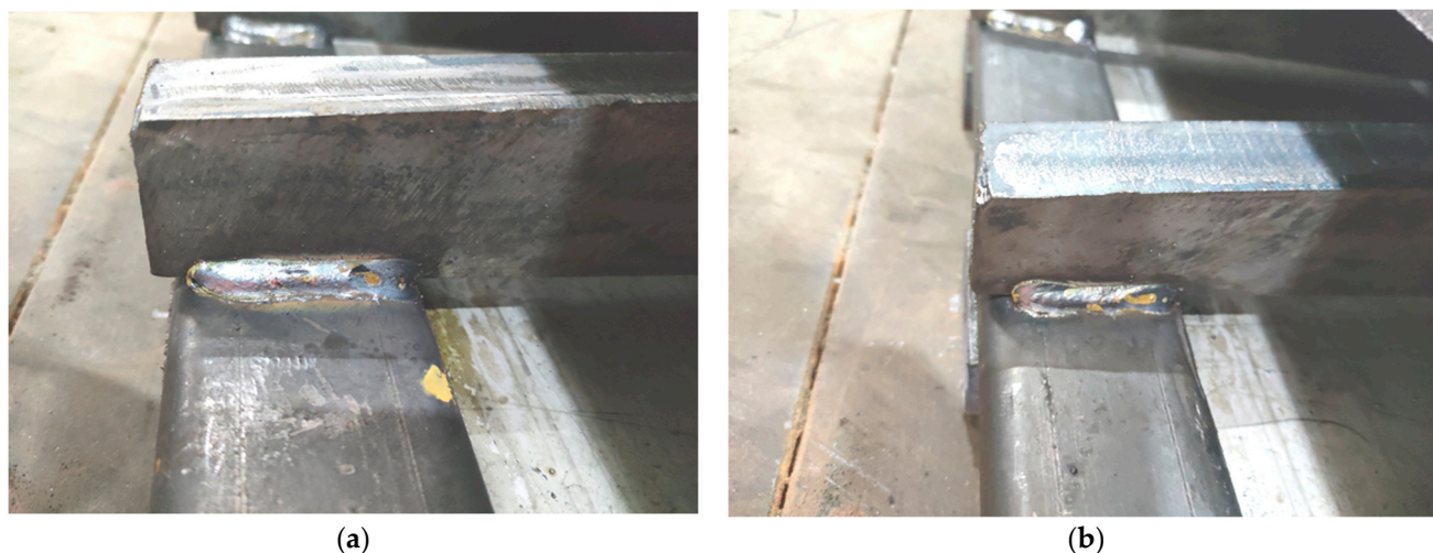
Figure 25. Welds of steel groove and support system: (a) From top to bottom in Figure 22b, Below the third teeth, (b) Below the fourth teeth.
