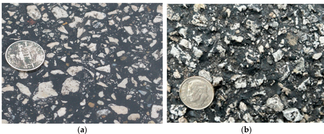
Figure 7. Close-up views of chip seal surfaces. (a) Slippery surface; (b) Rough surface.
