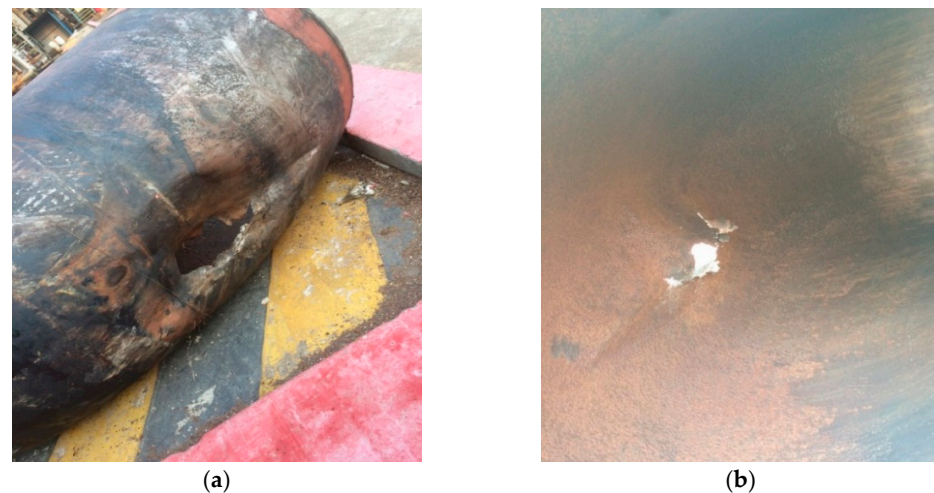
Figure 1. Leakage occurring in the elbow: (a) outside view; (b) inside view.
