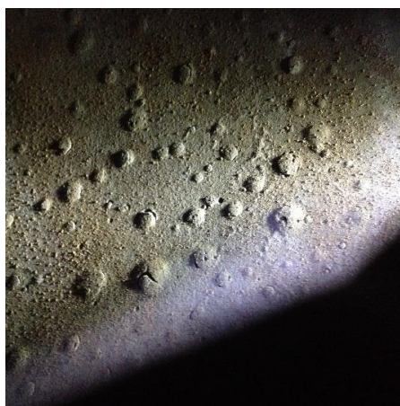
Figure 1. Blistering in internal surface.
