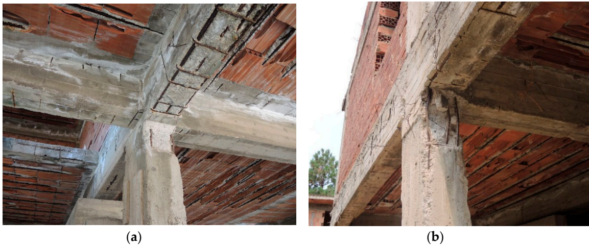
Figure 16. Run #9, 62.4 mm—1.69%: Concrete spalling, core crushing, and reinforcement buckling at the top of column c6 (a) and c13 (b).
