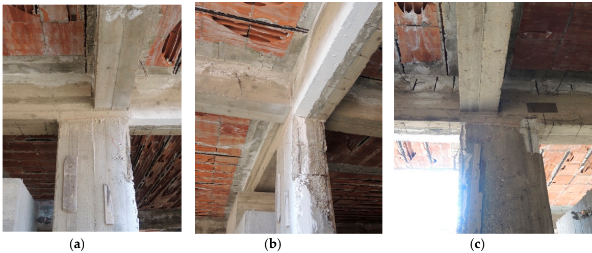
Figure 17. Run #9, 62.4 mm—1.69%: Damage at the top of column c5. Front (a), side (b) and back (c) view.
