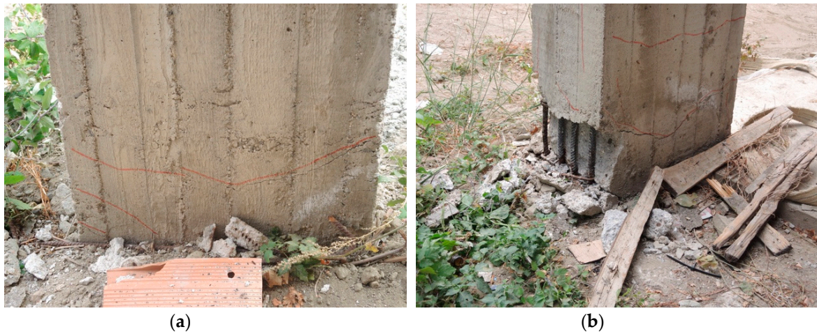
Figure 19. Run #9, 62.4 mm—1.69%: Flexural cracking pattern and failures at the base of columns c4 (a) and c18 (b).
