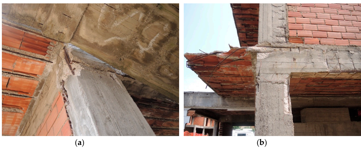
Figure 21. Run #9, 62.4 mm—1.69%: Joint damage at the top of column c14 (a) and c8 (b).
