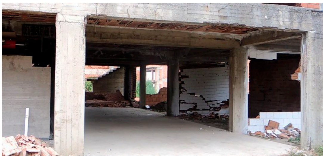
Figure 15. Run #9, 62.4 mm—1.69%: Infills parallel to the test direction fully collapsed.
