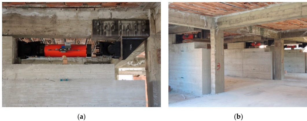
Figure 9. Actuation detail (a) and overview of the test setup (b).
