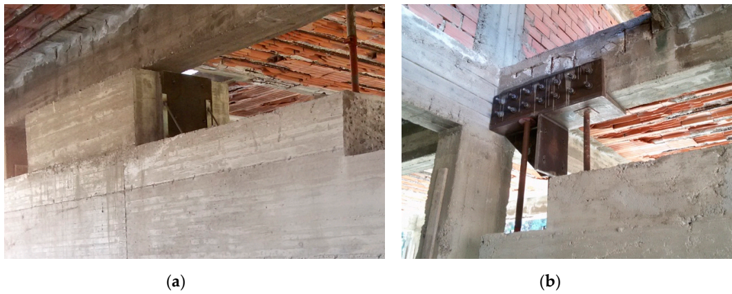
Figure 8. Steel element connections for the actuators: On the reaction wall (a) and on the frame first floor beam (b).
