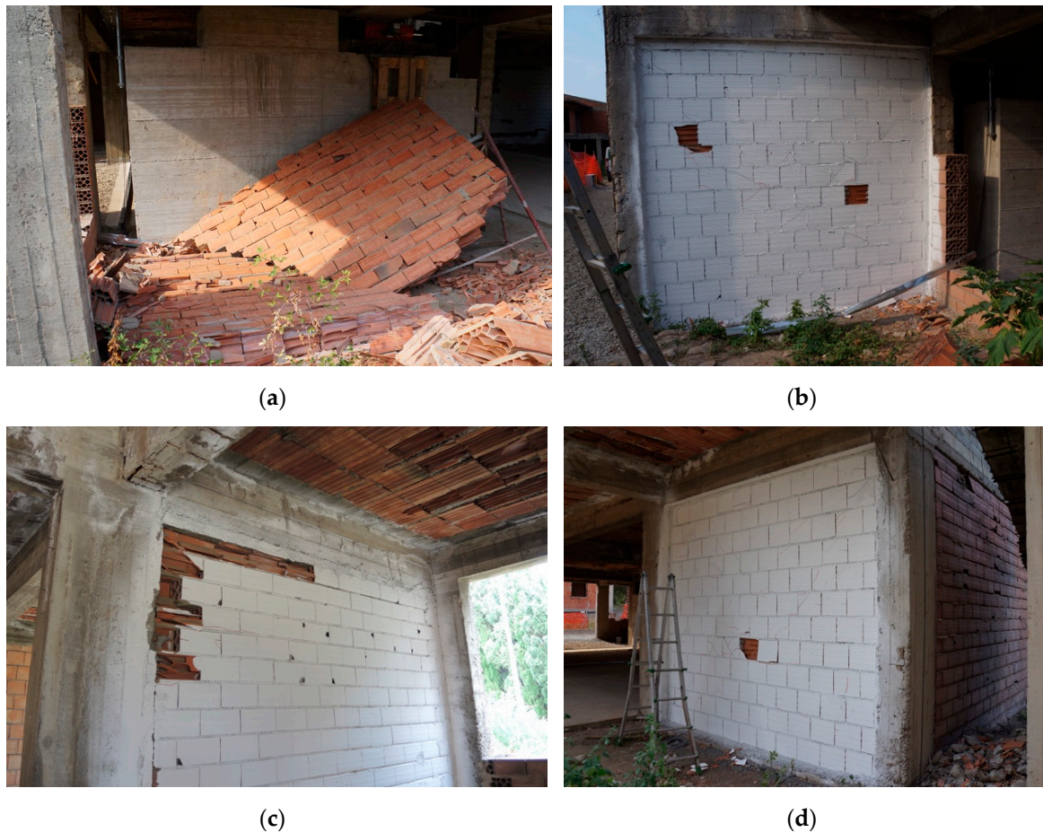
Figure 13. Infill damage at run #4, 9.6 mm—0.26%: Infill i5 (a); infill i3 (b); infill i10 (c); infill i11 (d).
