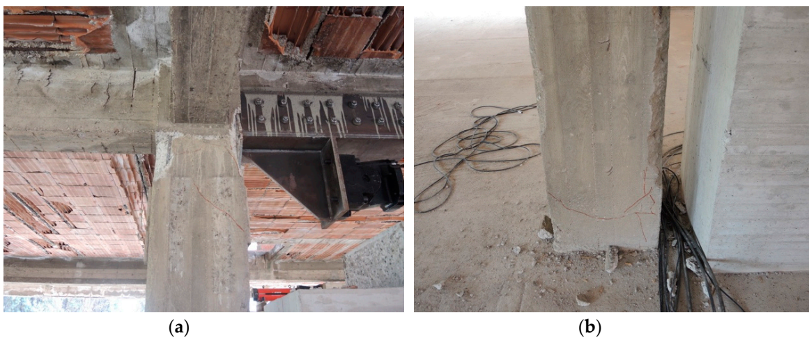
Figure 18. Run #9, 62.4 mm—1.69%: Damage at the top (a) and at the base (b) of column c11.
