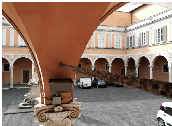
Figure 12. Internal courtyard of the Palazzo Arcivescovile. A total of 30 tie-rods are installed in the vaulted corridor surrounding it.
