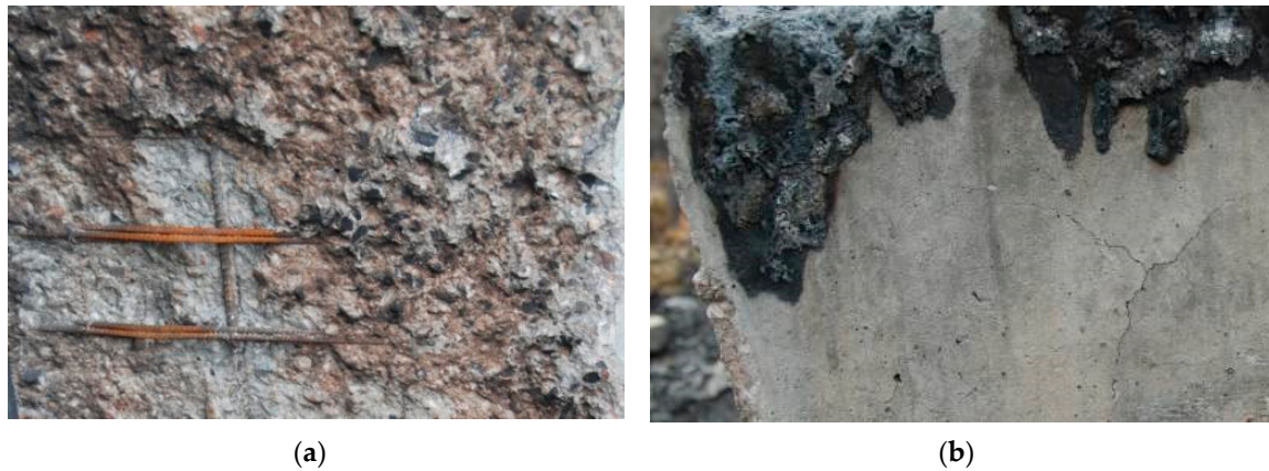
Figure 1. (a) Split and (b) cracking of concrete cover after firefighting.
