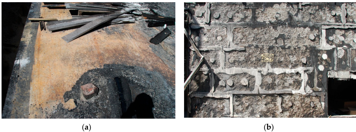
Figure 2. Concrete surfaces after fires: (a) top surface partially covered with watertight bituminous material, (b) vertical surface insulated with Styrofoam.
