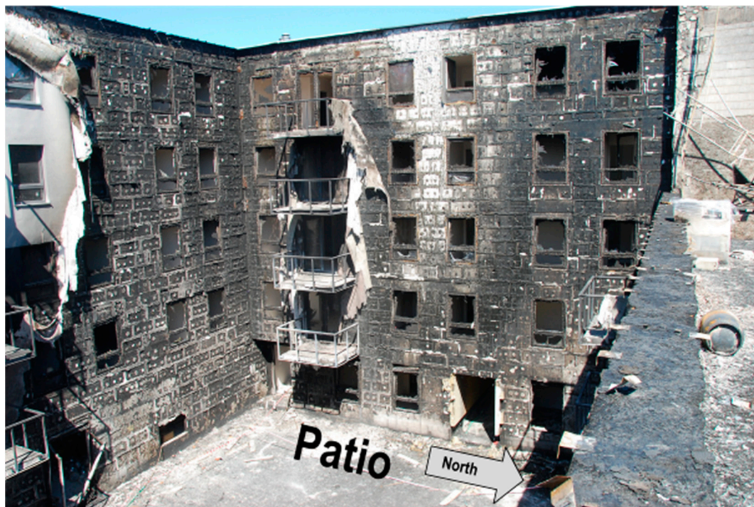
Figure 5. Façades after the fire.
