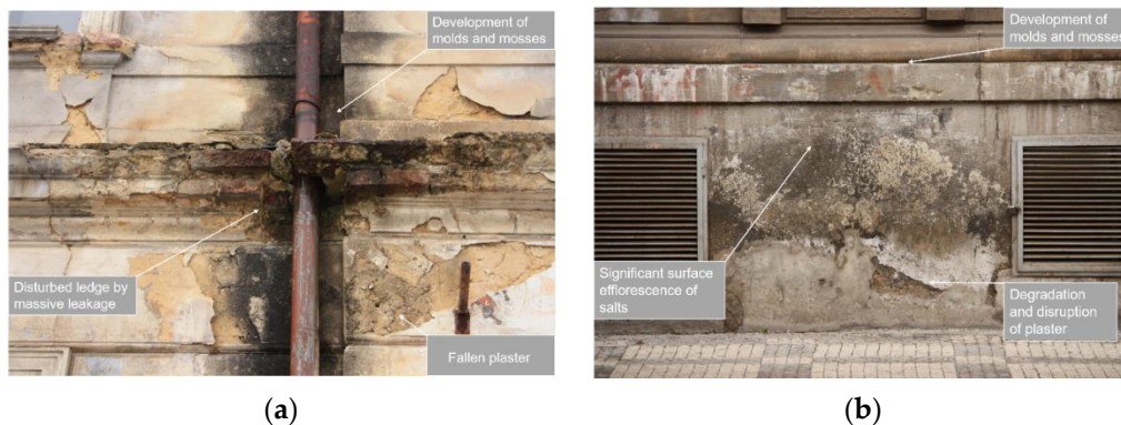
Figure 2. Images clearly showing the most common failures of structures from the second half of the 19th and the early 20th centuries caused by degradation processes initiated in these cases by the combination of moisture, an incorrect design solution and neglected maintenance. The following are clearly visible on images: (a) fallen plaster, damaged ledge by massive leakage, mold and mosses; (b) degradation and disruption of plaster, significant surface efflorescence of salts, mold and mosses.
