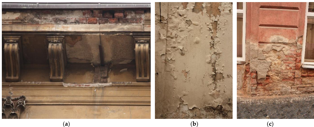
Figure 9. Examples of non-structural failures caused by the effects of the external environment, especially the synergic effect of increased moisture levels and temperature, which are accompanied by chemical, mineralogical and biological processes in structures from the second half of 19th century and the start of 20th century: (a) damage of the ledge and its surface finishes, visible salt efflorescence; (b) closed and open blisters in the surface layers due to their low diffusion permeability; (c) extensive damage to the plinth part caused by the long-term effect of humidity and salts.
