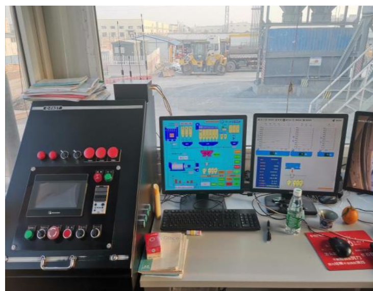
Figure 2. Data acquisition equipment in control room of mixing plant.
