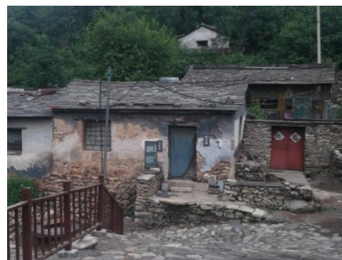
Figure 3. Stone foundation of a building in Shuiyu village, Fangshan district of Beijing City.
