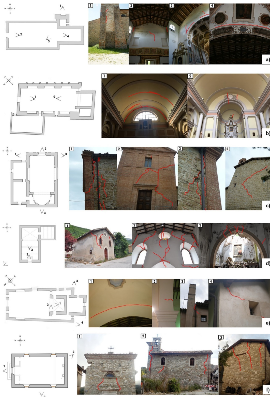
Figure 2. Main damages in: San Francesco Church in Montefortino (a), San Francesco Church in Sarnano (b), Sant'Anna Church in Camerino (c), Sant'Antonio Church in Ussita (d), Madonna of Valcora Sanctuary in Fiuminata (e), Santissimo Crocifisso in Arquata del Tronto (f).
