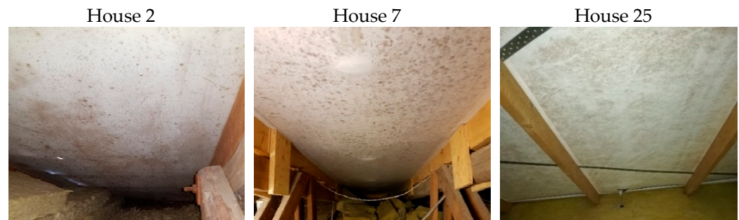
Figure 20. Mould growth in the attics of three test houses, namely houses 2, 7 and 25.
