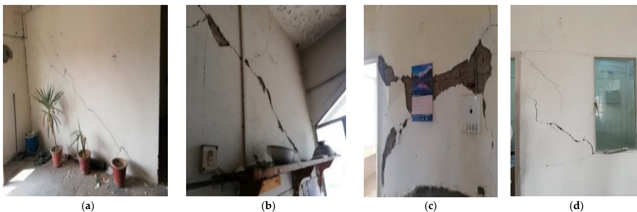
Figure 13. Cracks and damages observed in the infill walls (a–d) on the frame selected for analysis.
