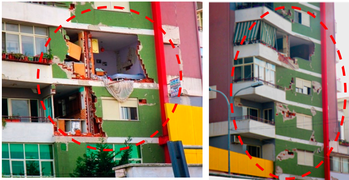
Figure 1. Collapse of unreinforced masonry facades of multi-story R/C buildings in Dures, Albania (26th November 2019, in-situ visit).
