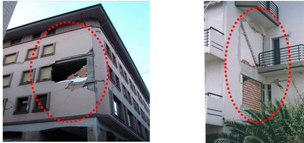
Figure 2. Collapse of unreinforced masonry facades of multi-story R/C buildings with thermo-insulation schemes located within the gap of a double wythe masonry panel. (Left) L'Aquila, Italy (2009), (right) Athens, Greece (1999) [3].
