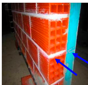
b) Flexural crack at mid-height both at the horizontal bed joint as well as at the XPS panel.
