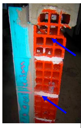
a) Debonding of XPS at the top and damage of top
