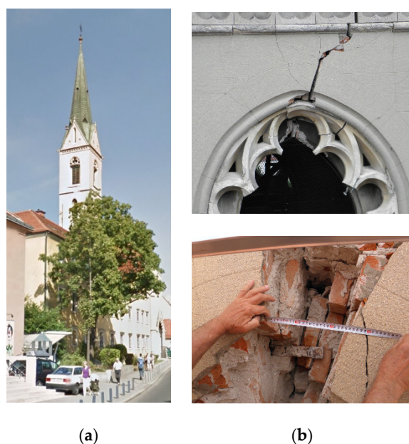
Figure 1. The bell tower of the church of St. Francis of Assisi on Kaptol in Zagreb: (a) bell tower in 2020; (b) some damage on the bell tower after earthquake 2020.
