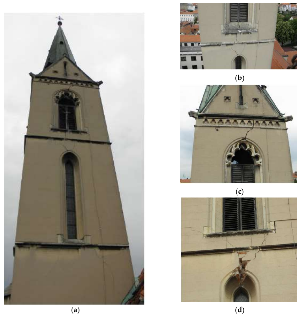
Figure 7. The cracks in the bell tower after the Zagreb earthquake on March 2020: (a) cracks in the east front wall; (b) the collapse of the lintel at the height of +27.26 m on the east wall; (c) characteristic cracks and damage of the lintel on the east wall; (d) characteristic cracks and damage to the lintel on the west front wall.
