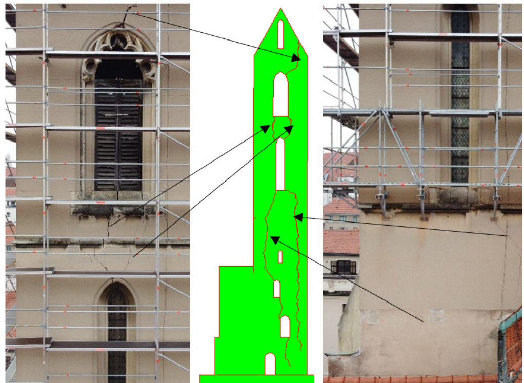
Figure 10. Comparison of cracks on the bell tower and on the numerical model.
