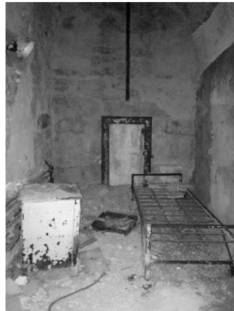
Figure 5. A cell at the Eastern Penitentiary Museum showing rough wall finishes.
