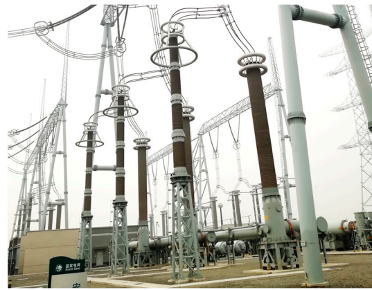
Figure 3. The 1000 kV surge arrester with supporting structure installed in an UHV electrical substation.
