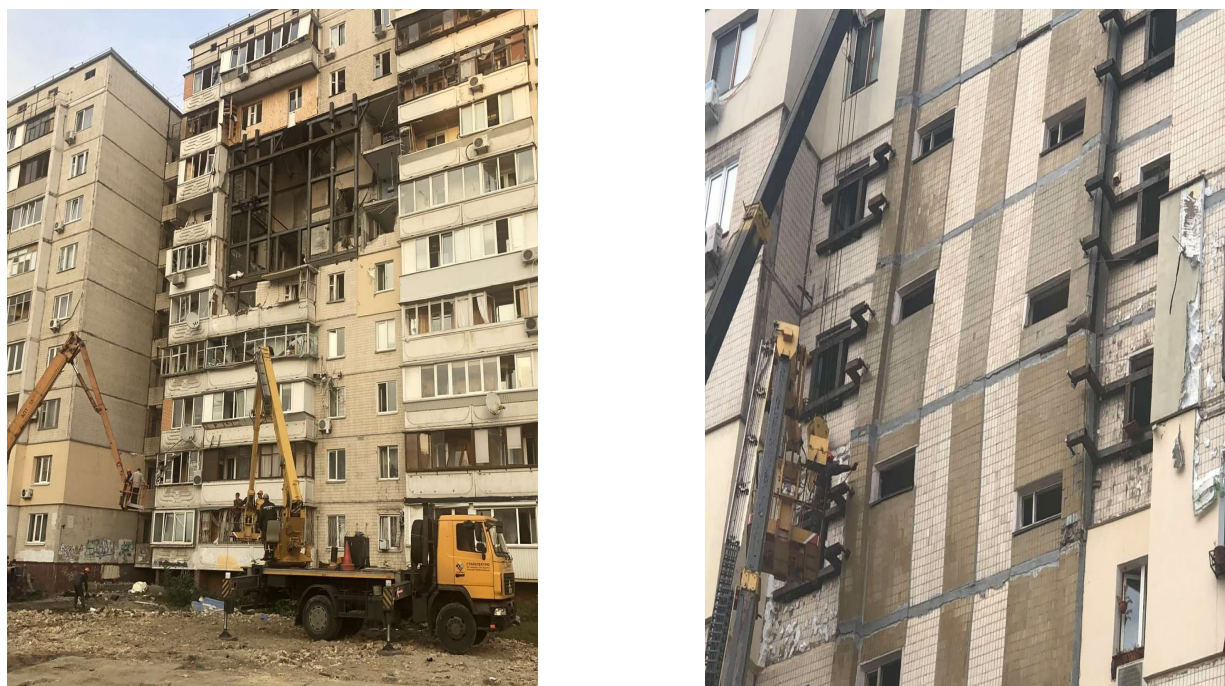
Figure 10. Urgent temporary stabilization of a large-panel building damaged as a result of a gas explosion (Kyiv city, S. Krushelnytska Street, June–October 2020).
