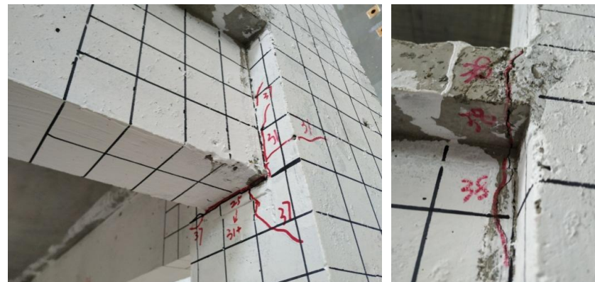
(b) The damage was aggravated at the beam-column joints
