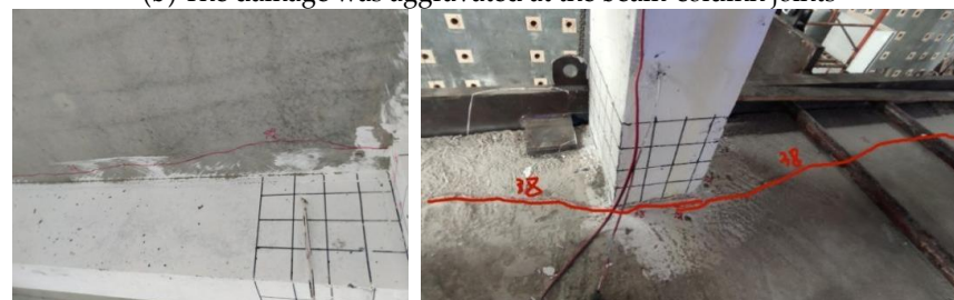
(c) The bottom of the first floor appeared horizontal through long cracks
