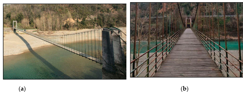
Figure 2. General views of the Ramello footbridge: (a) lateral view and (b) longitudinal view.
