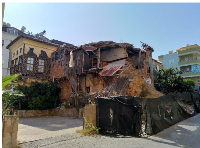
Figure 1. A deteriorated historic building in Turkey.
