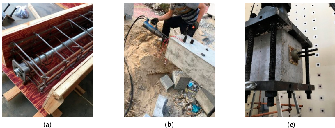
Figure 3. Post-tensioning tendon construction: (a) embedding corrugated duct; (b) prestress wire tensioning; (c) prestress wire anchorage.
