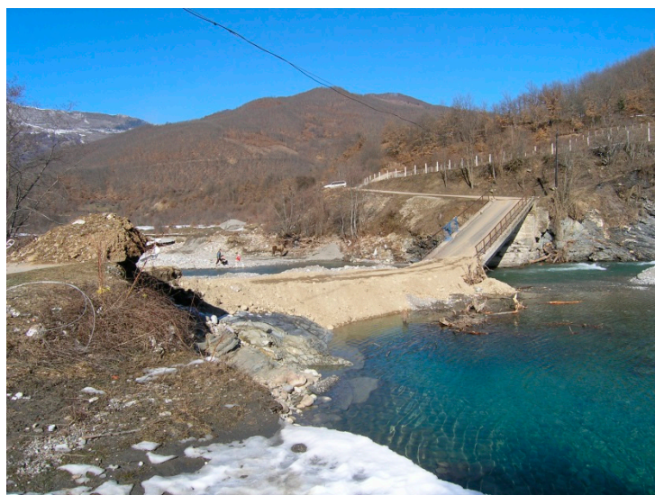
Figure 25. The Novsici bridge after the collapse.
