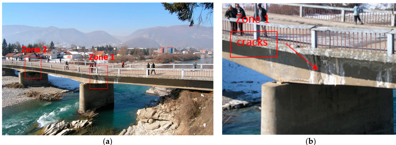
Figure 5. (a) The bridge after the settlement of the river pier and (b) cracks in zone 1.
