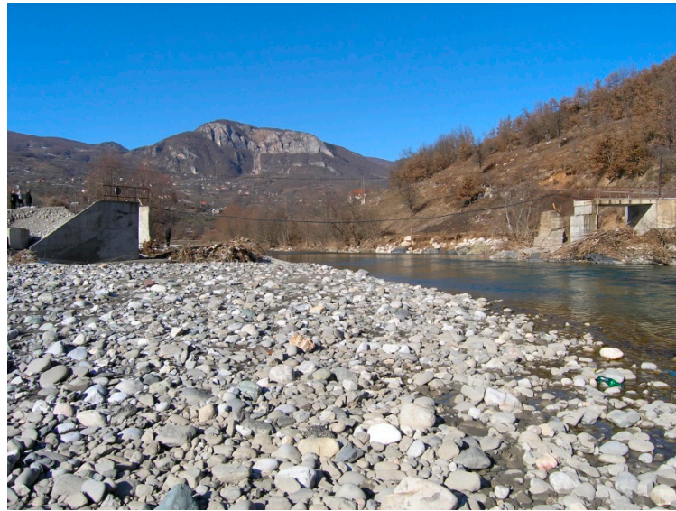
Figure 23. The Seoca bridge after the collapse.
