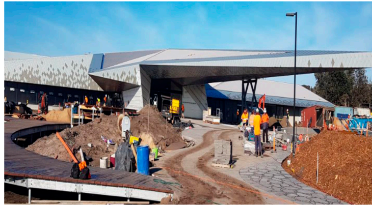
Figure 3. Cantilevered Roof and Box Gutters of Builder C3 (Adapted from Phillip Island Nature Parks [41]).
