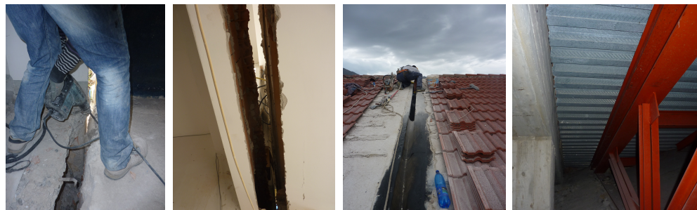
Figure 3. Details of the structural joints upgraded during the 2012 interventions (from left to right): increment of the distance between floor slabs; effective distance between floor slabs visible after the interventions; waterproof layer on the joint between two roof slabs; corrugated steel sheet between adjacent buildings A and C under the joint (photo courtesy of R. Amici).
