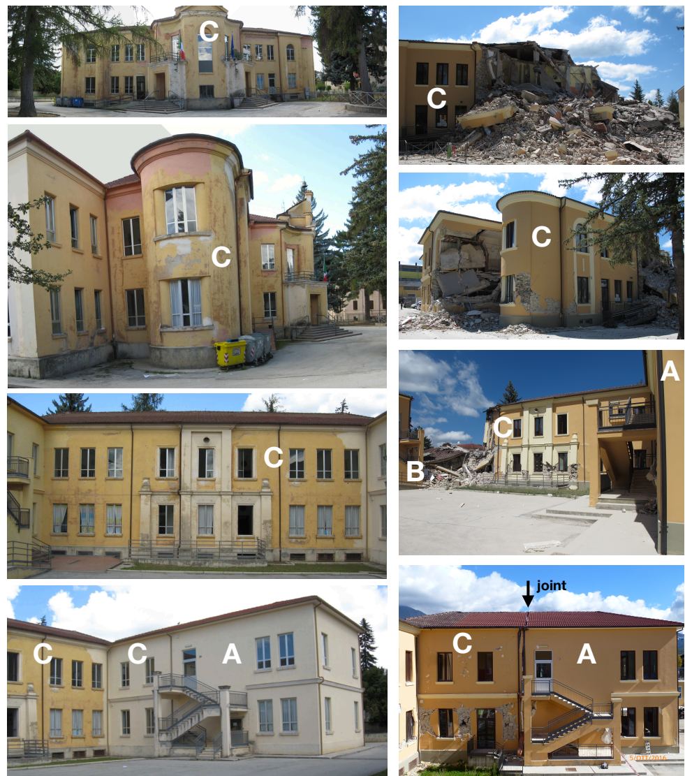
Figure 2. Views of the buildings before (left) and after (right) the 24 August 2016 earthquake; the letters refer to the nomenclature of the buildings reported in Figure 1b. The photographs on the left were taken prior to the 2012 interventions.
