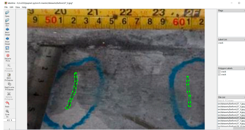
Figure 10. The crack data annotation.
