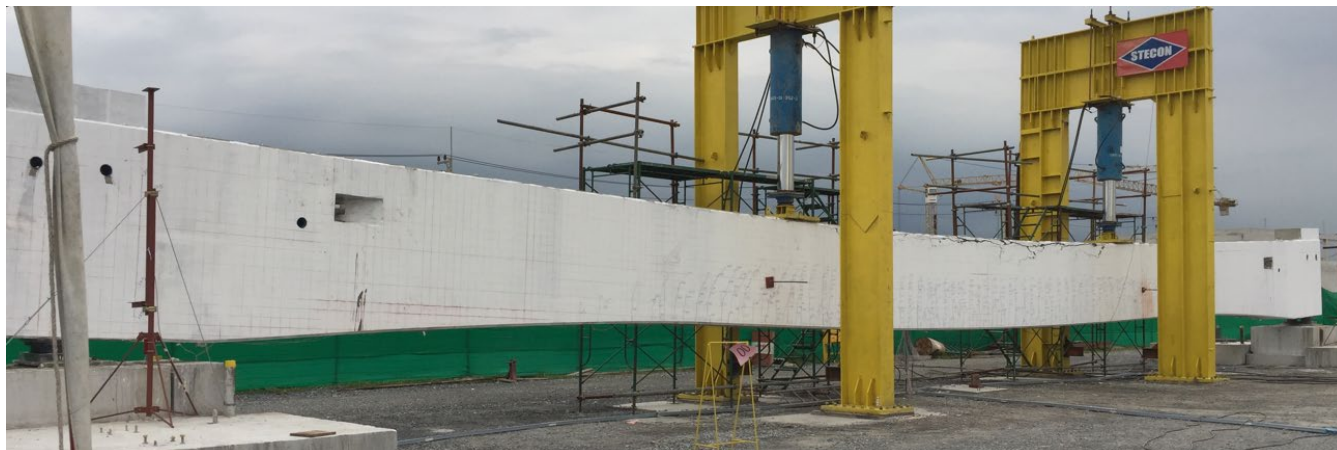
Figure 51. Ultimate failure of specimen SP-2.
