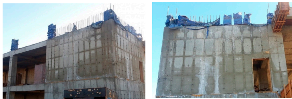
Figure 4. Frozen concrete structure of apartment building in November 2019 (average temperature was -9.6\text{ }^{\circ}\text{C} ).
