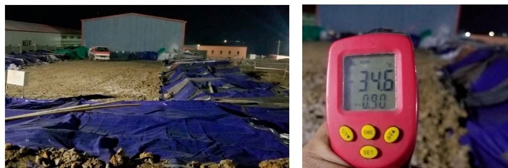
Figure 5. Concrete work of foundation executed in December 2019 (outside temperature was -34.6\text{ }^{\circ}\text{C} ).
