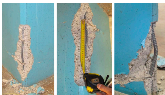
Figure 3. Damage to columns [1].
