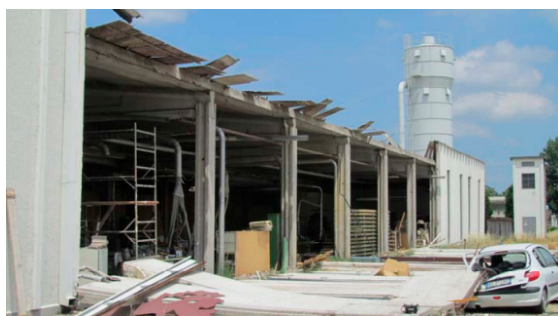
Figure 2. Collapse of infill panels [1].
