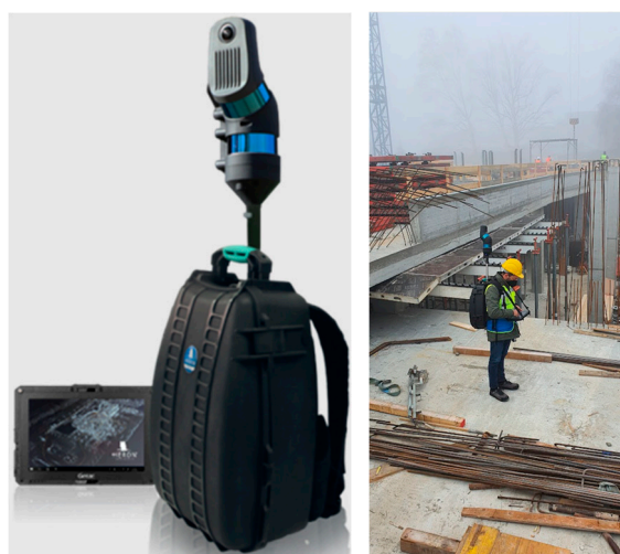
Figure 1. The wearable mobile mapping device ( left ) and its use during the monitoring phase at the construction site ( right ).
