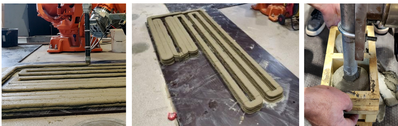
Figure 4. Printing process (left), printed wall section before covering with PE film (middle), and filling the cubes before compaction (right).
