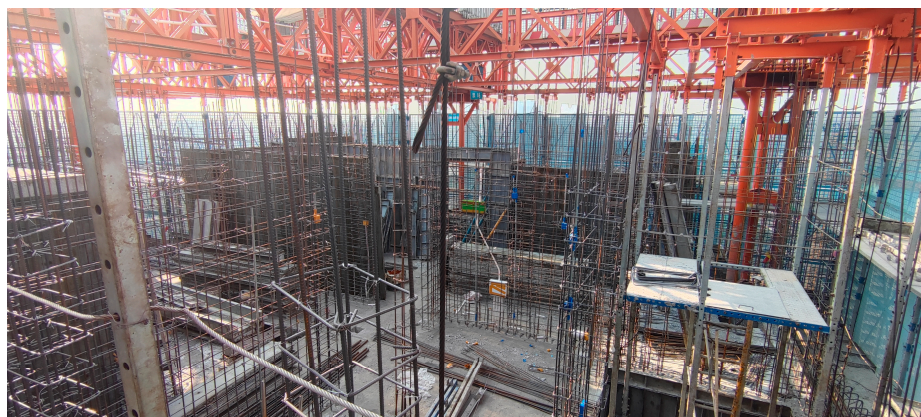
(c) Interior of building machine
