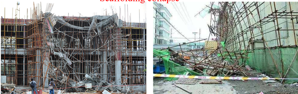
Figure 2. Construction accident-scaffold collapse case.
